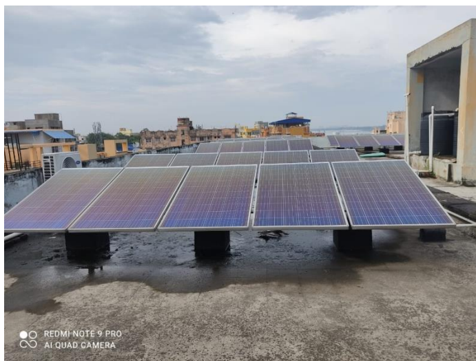
RPMC ROOF TOP WITH INSTALLED SOLAR PANNELS
