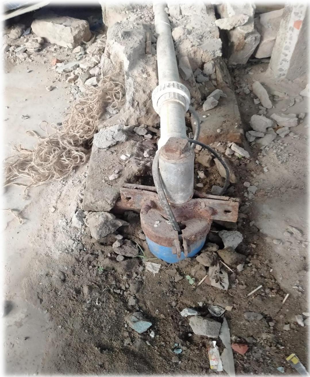
Bore well /Open well recharge
